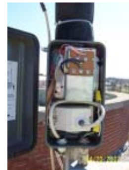
Transformer, furnace coil, etc., to generate spark
