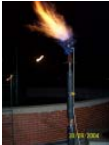
Waste Gas Burner
