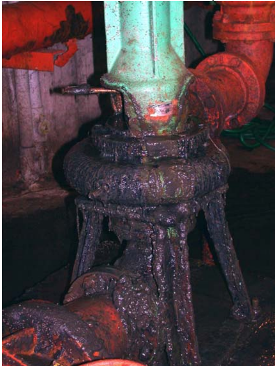
Poor Maintenance - Use of channel locks to hold in the packing of a return sludge pump, instead of performing required repairs. Sludge covered the floor, creating a health and safety concern.
