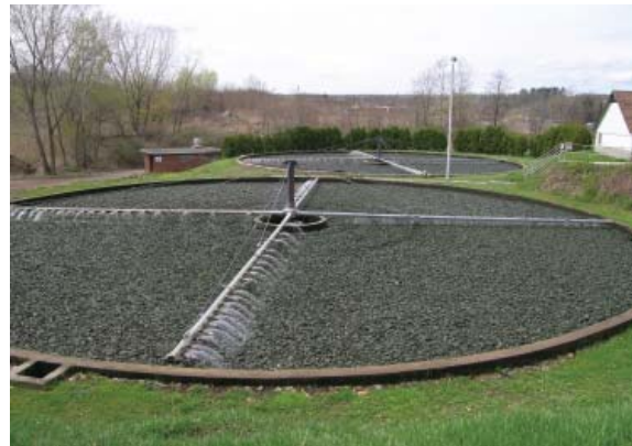
Many wastewater treatment facilities in New York are operating beyond their useful life expectancy.
