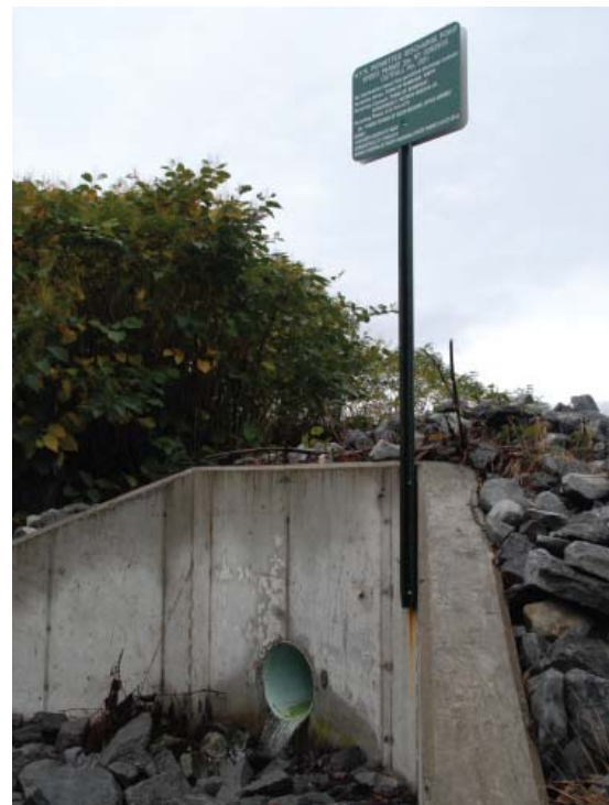
A wastewater treatment facility outfall. Clean water is discharged to our streams, rivers and lakes.
