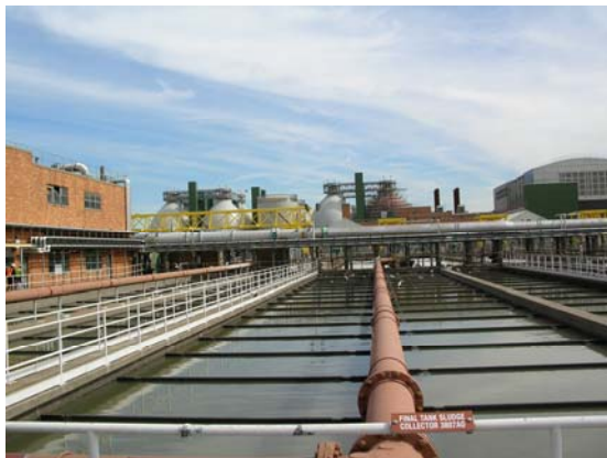
Final clarifier at Newtown Creek WWTP
