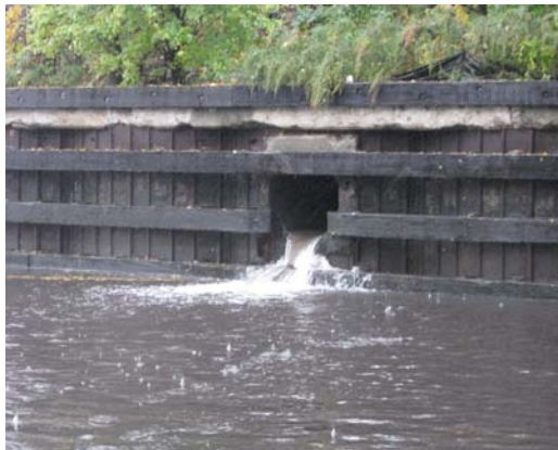
CSO on the Hutchinson River
