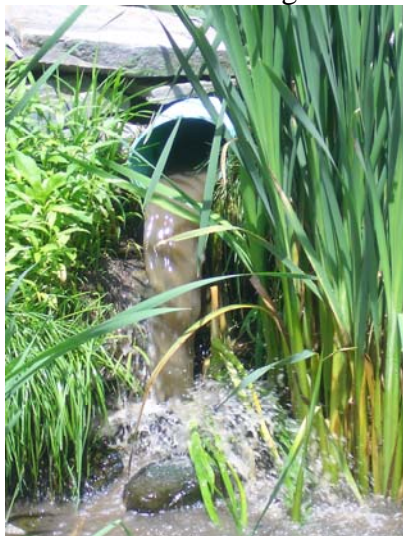
Discharge from Rushmore/Brigadoon Estates WWTP
