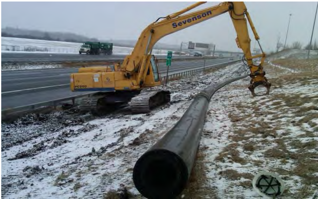
Slurry Pipeline Along 690
