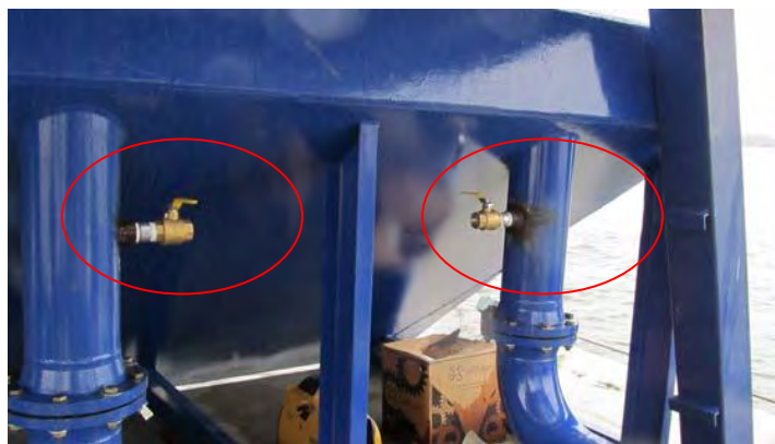
Sample Ports on Vertical Riser Before Slurry Enters The Diffuser Plate
