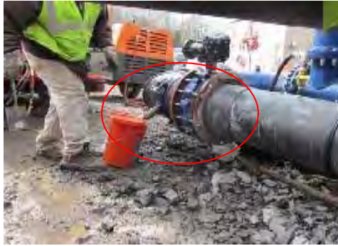
GAC/Sand Slurry Mix Line Sample Port
