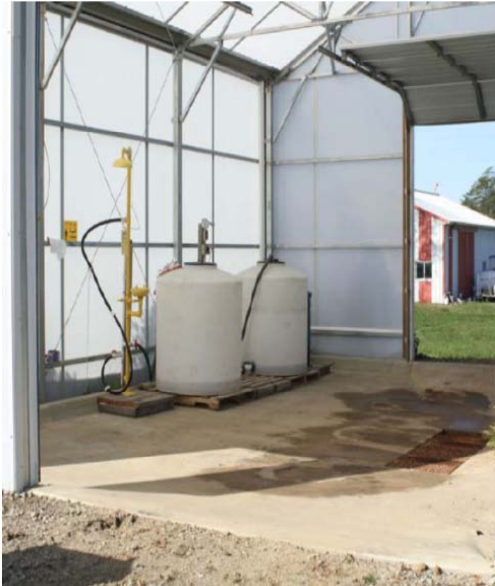
Figure 1: Agricultural Pesticide Handling Facility Installed at Starkie Family Farms, Cutchogue
