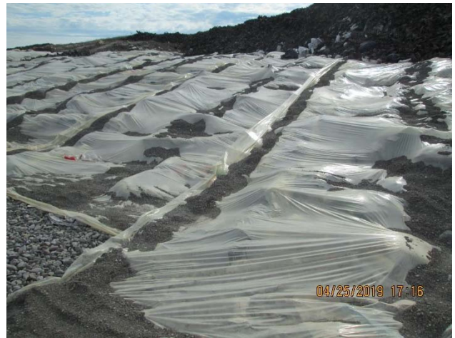
High Acres Landfill - Enviro Cover deployed with stone ballast
