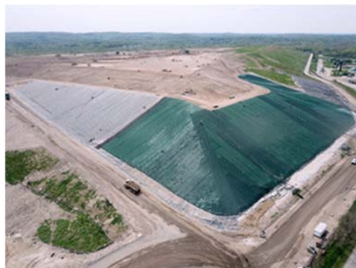
High Acres Landfill – engineered soil cover and geomembrane cover systems
