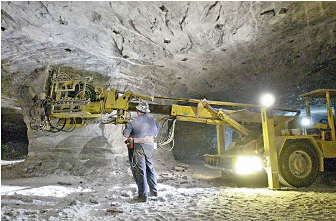
Worker installing roof bolts at Cargill's Lansing Mine. Photograph by Simon A. Wheeler, Elmira Star Gazette 2002, copyright 2004.
