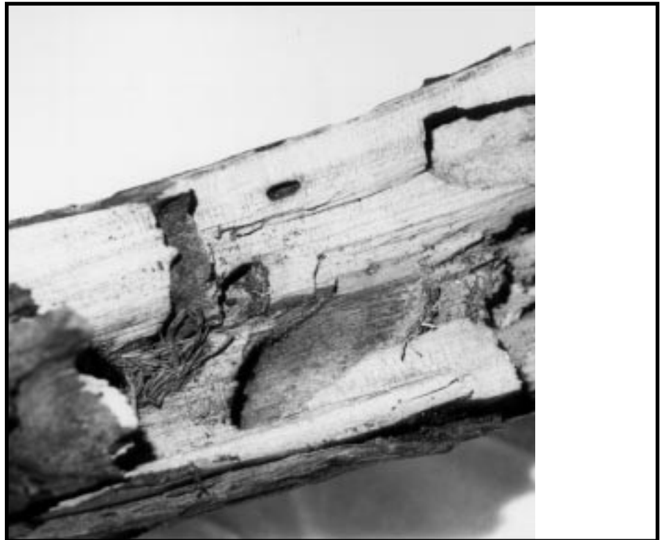
Fig. 5 Extensive damage to the interior of a large branch. The Gallery is 0.5" wide.
