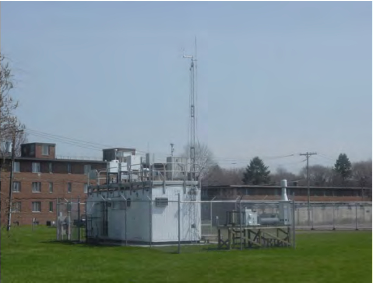
Rochester RG&E Substation Yarmouth Road Rochester, NY 14610
