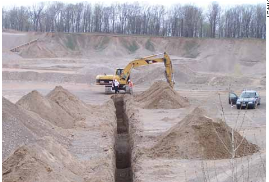
Excavating a test trench in the central part of the mine to try and locate the source of contamination.
