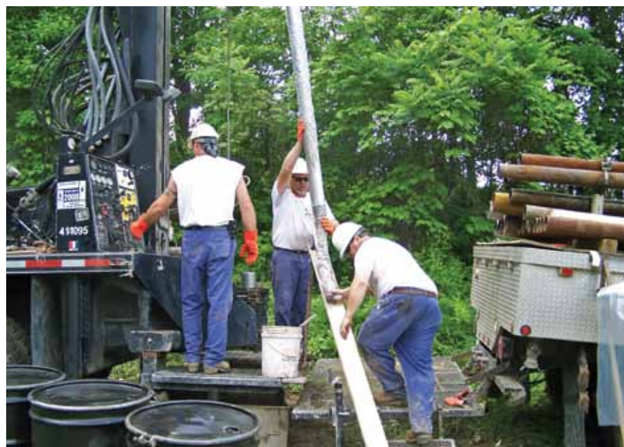
Drillers retrieve soil samples from an area north of the sand and gravel pit prior to installation of a groundwater monitoring well.
