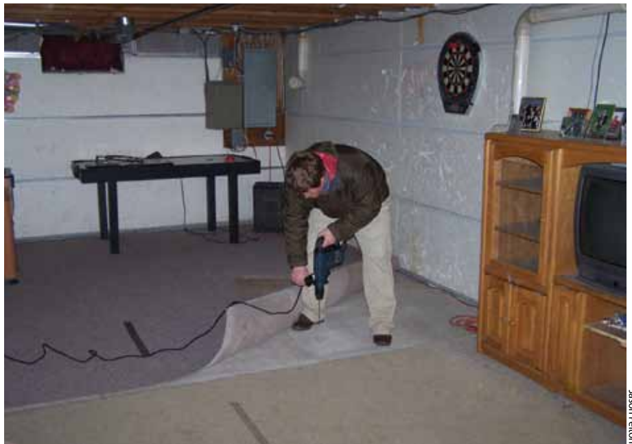
DEC contractor drilling a hole in the basement floor to determine if a depressurization system (used to alleviate vapor intrusion) is properly working.
