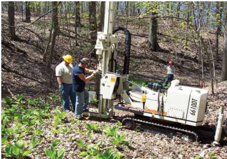
Workers sample the soil and install a groundwater monitoring well near Modock Road Springs.
